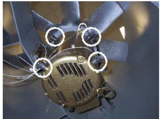
Figure 4: Motor bearing housing transducers
