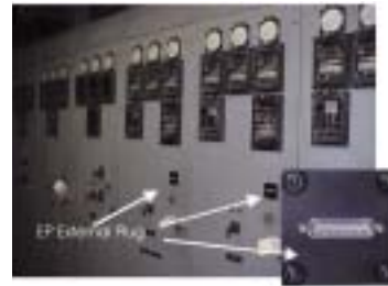
A typical motor control cabinet with the external plug shown, enabling safe on-line motor testing with the Explorer.
